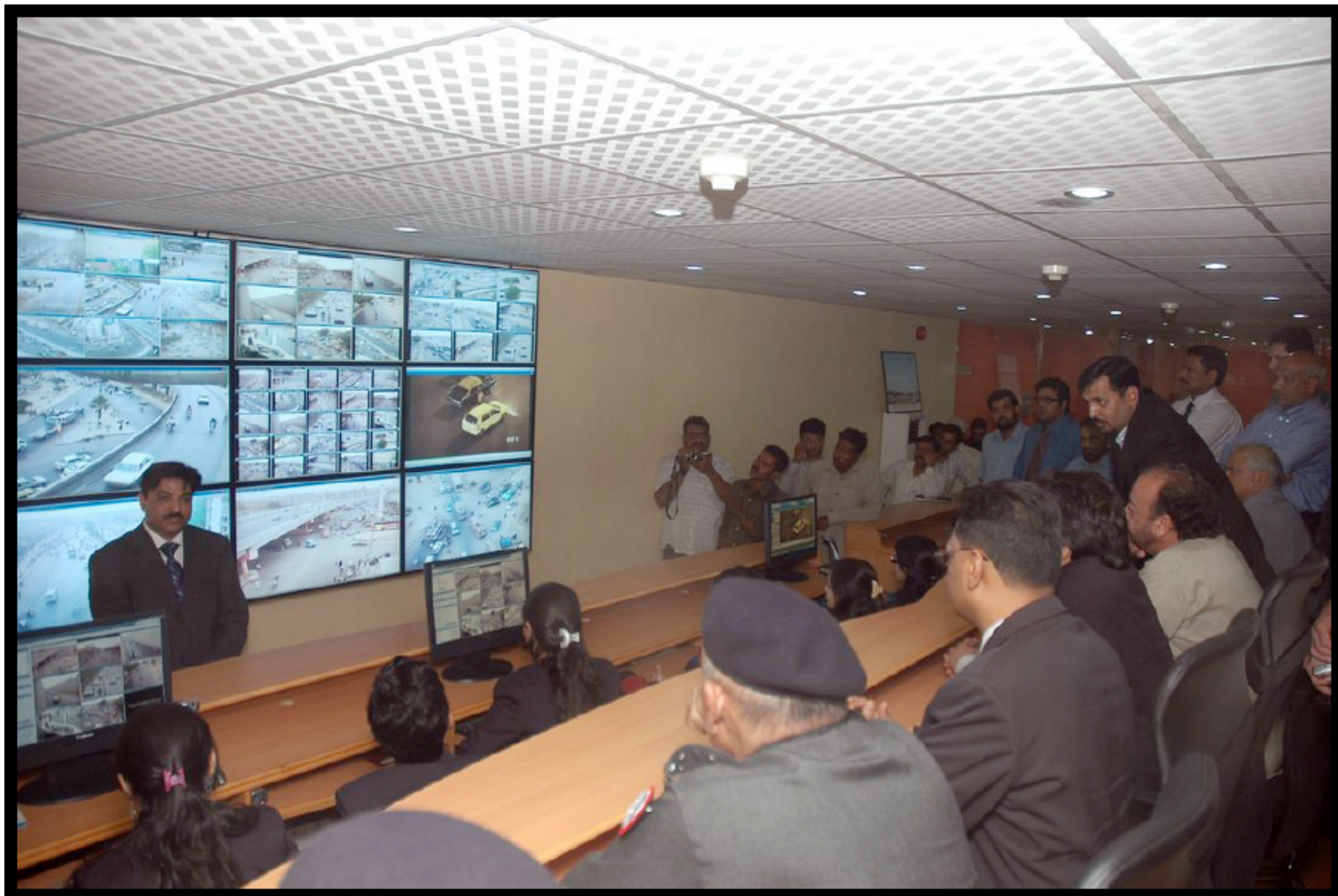
Video Wall Installed in Karachi, Pakistan 2008
